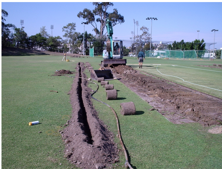
Figure 17: - Irrigation line 3m from Wicket Block
